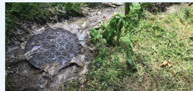
Wastewater manhole overflowing during heavy rain due to stormwater infiltration.
